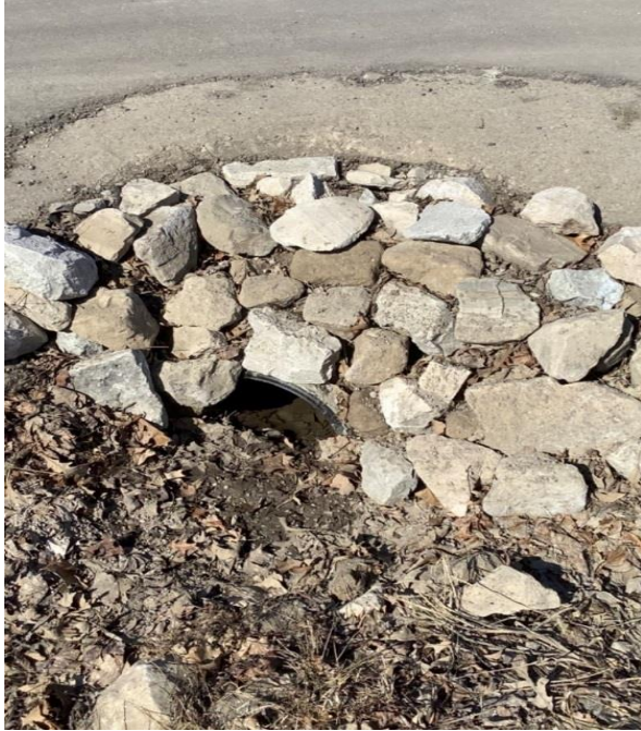
3697 Turner Road – 300mm diameter CSP pipe culvert with no observed deformation and rusted. Approximately 70% of this pipe was observed to be blocked with debris. The headwall consists of concrete and stone.
