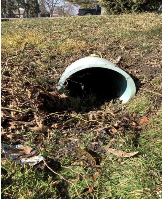
3860 Woodward Boulevard – 300mm diameter PVC pipe culvert that is in good condition with no observed deformation. Approximately 10% of this pipe was observed to be blocked with debris. No headwall was observed for this culvert.
