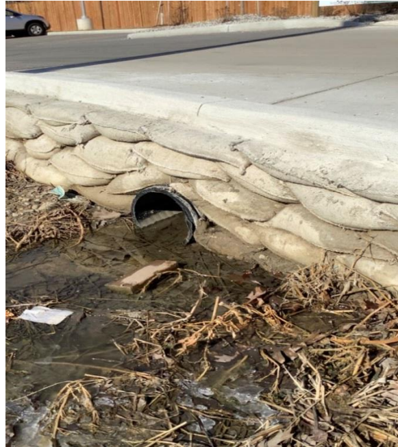
1840 Division Road – 250mm diameter HDPE pipe culvert that is in excellent condition with no observed deformation. There was no blockage of this pipe and the undamaged headwall is constructed with jute bags.
