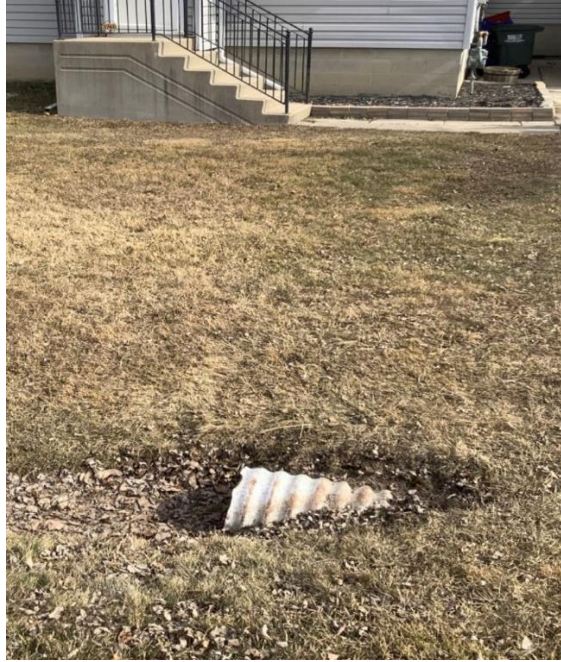
3726 Riberdy Road – 375mm diameter CSP pipe culvert with no observed deformation but rusted. Approximately 20% of this pipe was observed to be blocked with debris. No headwall was observed for this culvert.
