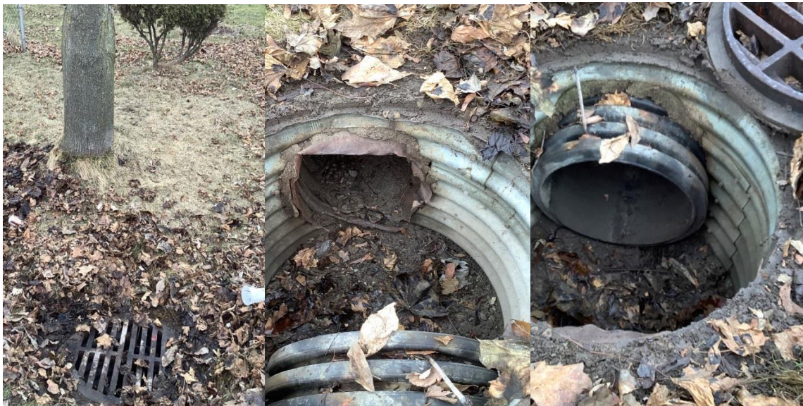
3791 Turner Road – An undamaged 600mm circular CSP catch basin observed. Two 375mm pipes (one is CSP and the other is HDPE) found connected to this catch basin. The 375mm CSP pipe is deformed and rusted. There was no discharge pipe observed connecting to this catch basin. There is approximately 10% blockage in the 375mm CSP pipe.
