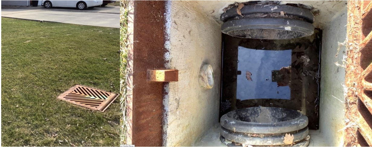
3778 Byng Road – An undamaged 600mm x 600mm square concrete catch basin observed. Two 375mm HDPE pipes were found connected to this catch basin with no deformation and no blockage within the pipes. A 100mm PVC discharge pipe is shown connected to the catch basin from private property.
