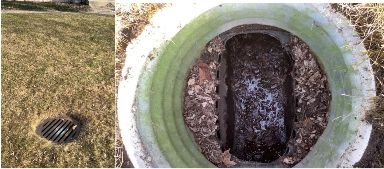
3873 Byng Road – An undamaged 450mm circular HDPE catch basin was observed. Two 300mm HDPE diameter pipes found connected to this catch basin with no deformation. There is approximately 10% blockage in both the 300mm diameter pipes. There was no discharge pipe observed connecting to this catch basin.
