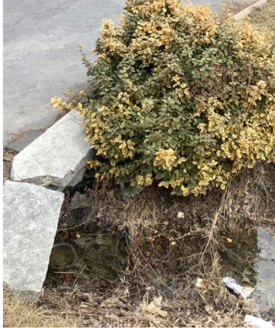
3923 Riberdy Road – 375mm diameter CSP pipe culvert with no observed deformation and rusted. Approximately 40% of this pipe was observed to be blocked with debris. The headwall is a mix of the asphalt driveway and the stone resting on top of it.
