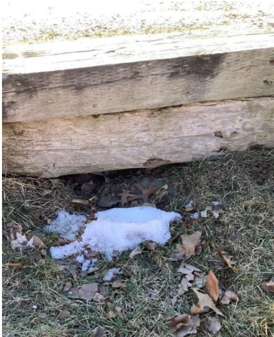
3949 Woodward Boulevard – Unknown CSP pipe diameter that was observed to be rusted. Approximately 90% of this pipe is blocked with debris and the headwall is made of pressure treated wood that is in good condition.
