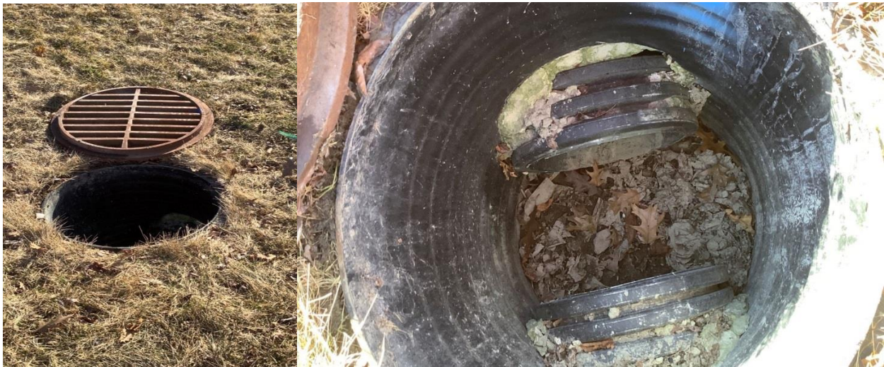
3750 Bliss Street – An undamaged 600mm circular plastic catch basin was observed. Two 375mm HDPE diameter pipes found connected to this catch basin with no deformation and no blockage within the pipes. There was no discharge pipe observed connecting to this catch basin.
